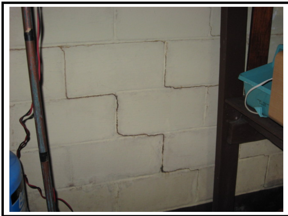
4. Step cracks in basement.
