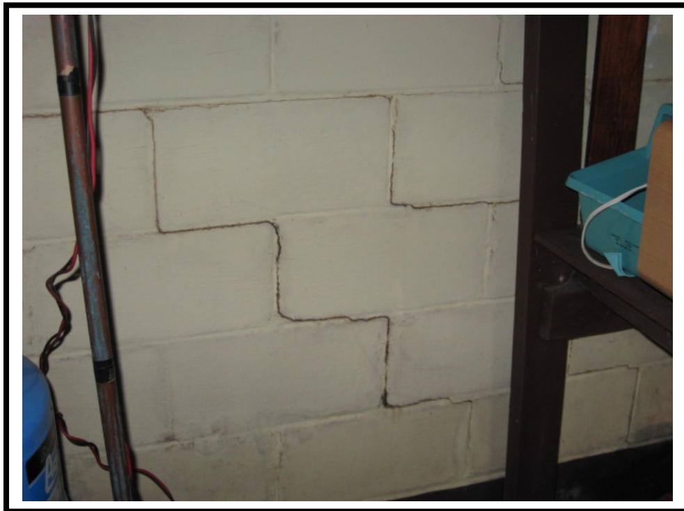
4. Step cracks in basement.
