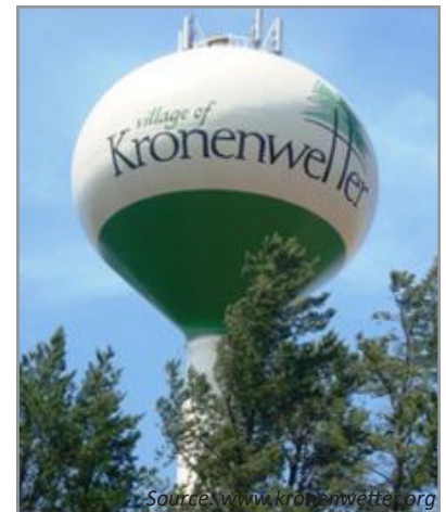
Source: www.kronenwetter.org Water towers are an element of a public water utility's infrastructure.
