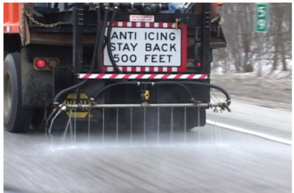
(Anti-icing - A snowplow applying salt brine to a road prior to a winter storm.)
