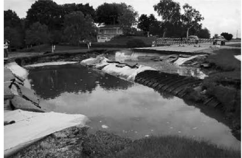
An example of serious damage to road infrastructure from Wisconsin's storms of summer 2008.
