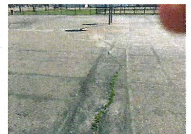
EXISTING PAVEMENT CRACKING
