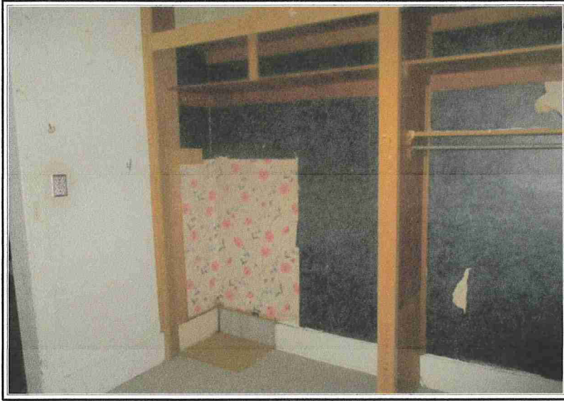
NO CLOSET DOORS DOWN
