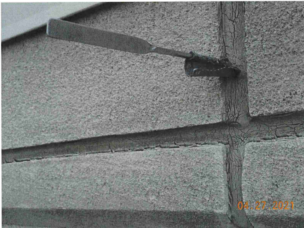
Photo #64: The spatula is slid into the deteriorated caulk joint about 3". Failed joints could be the cause of leakage at the window heads.
