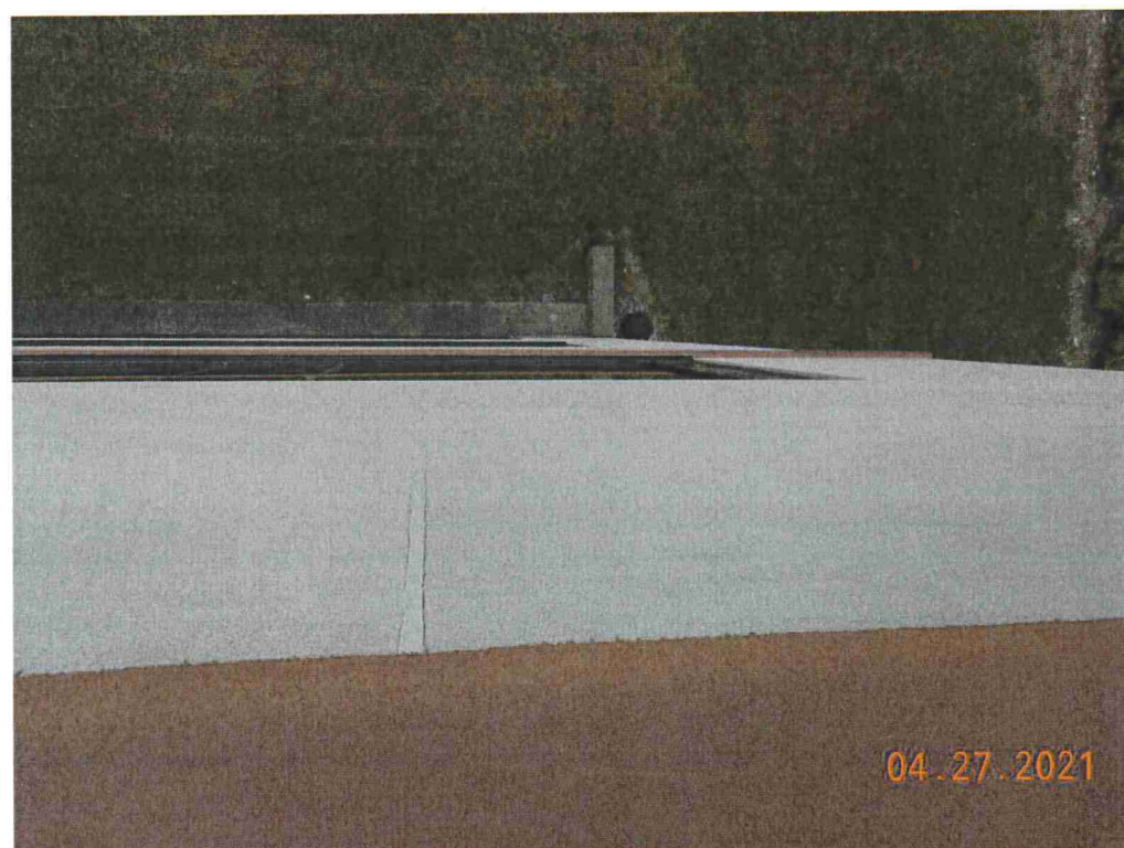
Photo #70: This is the west elevation, north end where the office is that leaked below. There is no flashing protruding from the window head and the joints in this area are still mortared with cracks.
