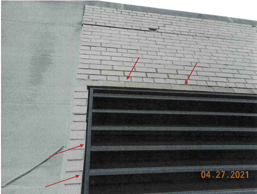
Photo #41: Grind out and caulk that joint above the new brick, directly above the louver. Seal the exterior of the louver frame to the brick.
