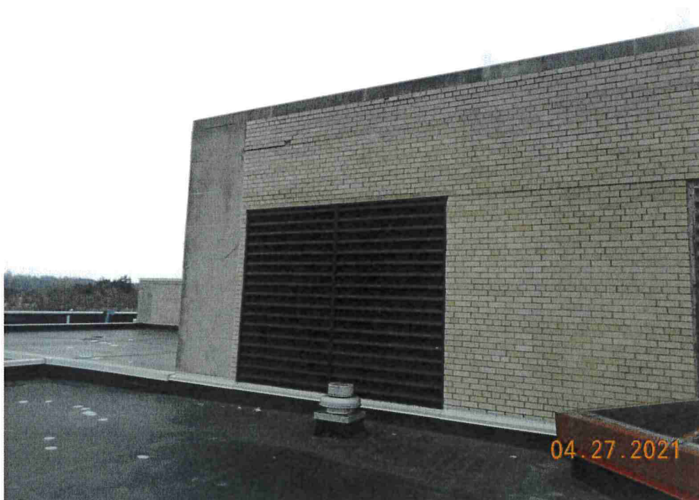
Photo #40: Northeast corner, new louver location. This wall it's self has taken a beating and needs some attention.
