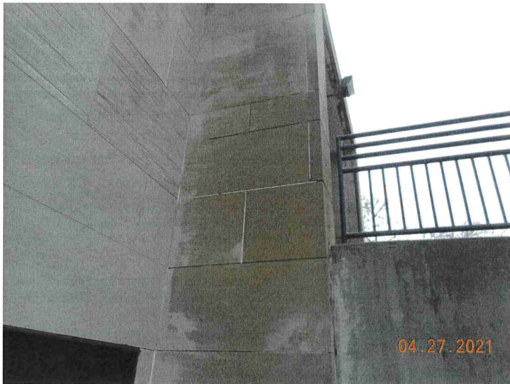
Photo #72: North wall of the west entrance needs all joints attended to.
