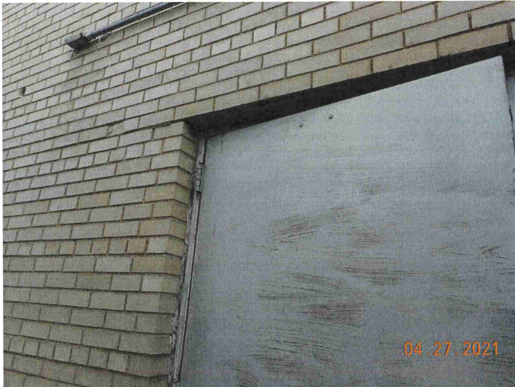
Photo #43: Replace the seals at the hollow metal door frames.
