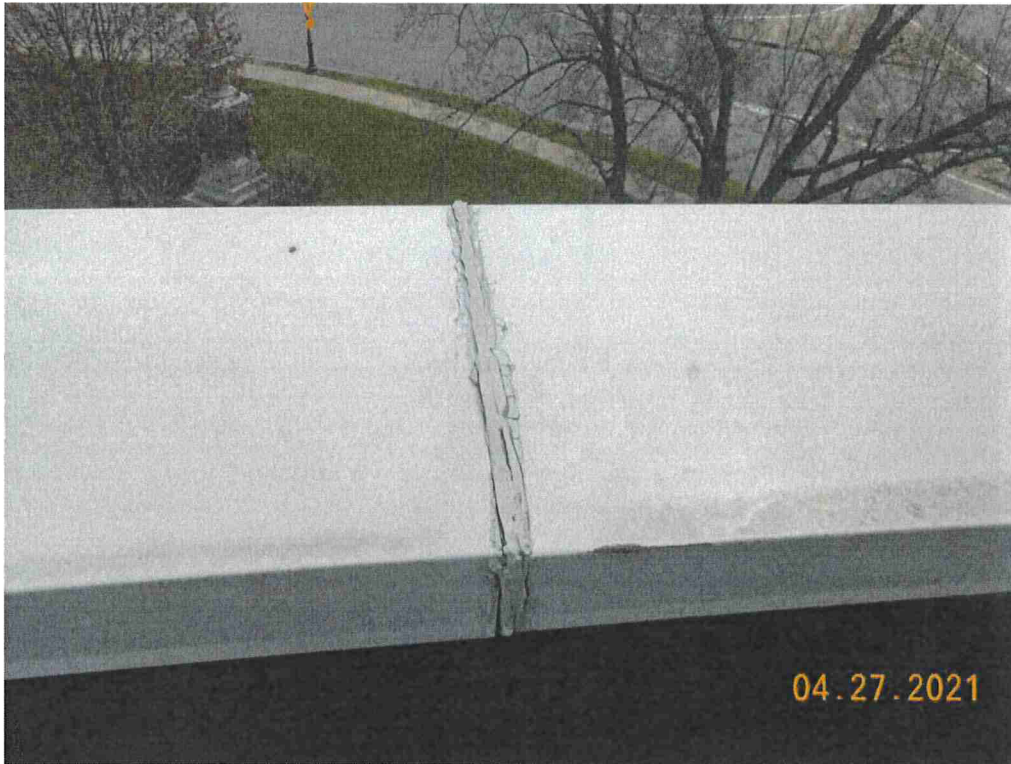
Photo #61: I would recommend a procured silicone boot bedded in sealant at the coping splice joints, not just sealant.
