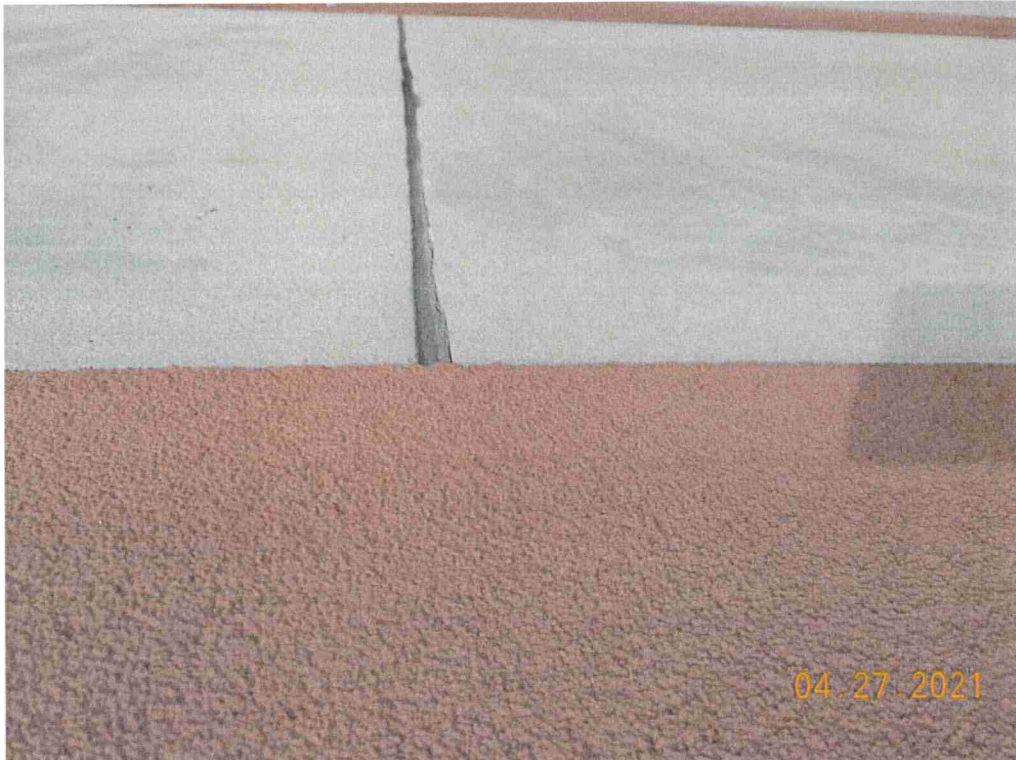
Photo #63: Vertical joint at the upper floor is caulked, needs to be replaced.
