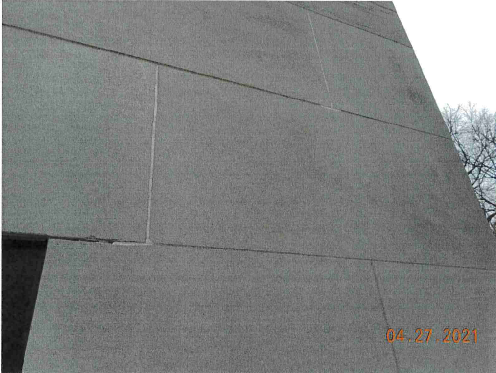
Photo #71: The lighter color mortar is replacement mortar and the bonding of it to the adjacent substrate isn't that good.
