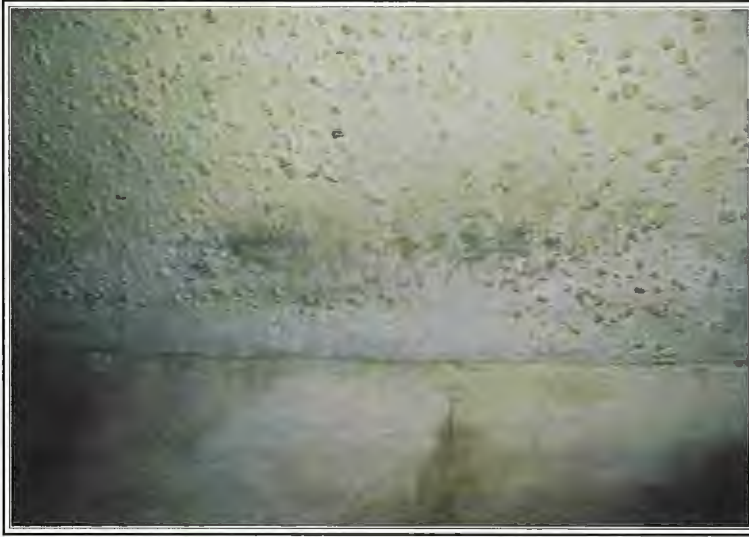
MOLD ON BEDROOM CEILING
