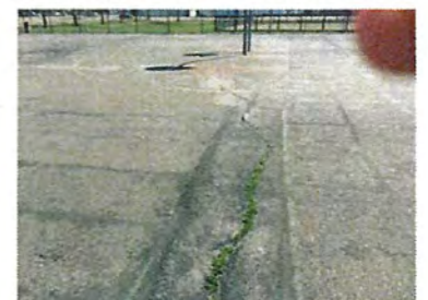
EXISTING PAVEMENT CRACKING
