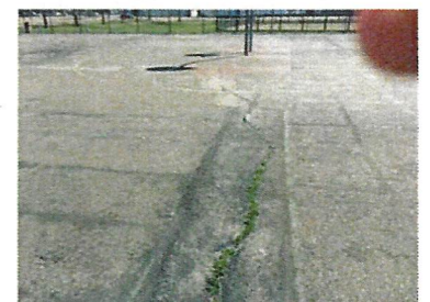
EXISTING PAVEMENT CRACKING
